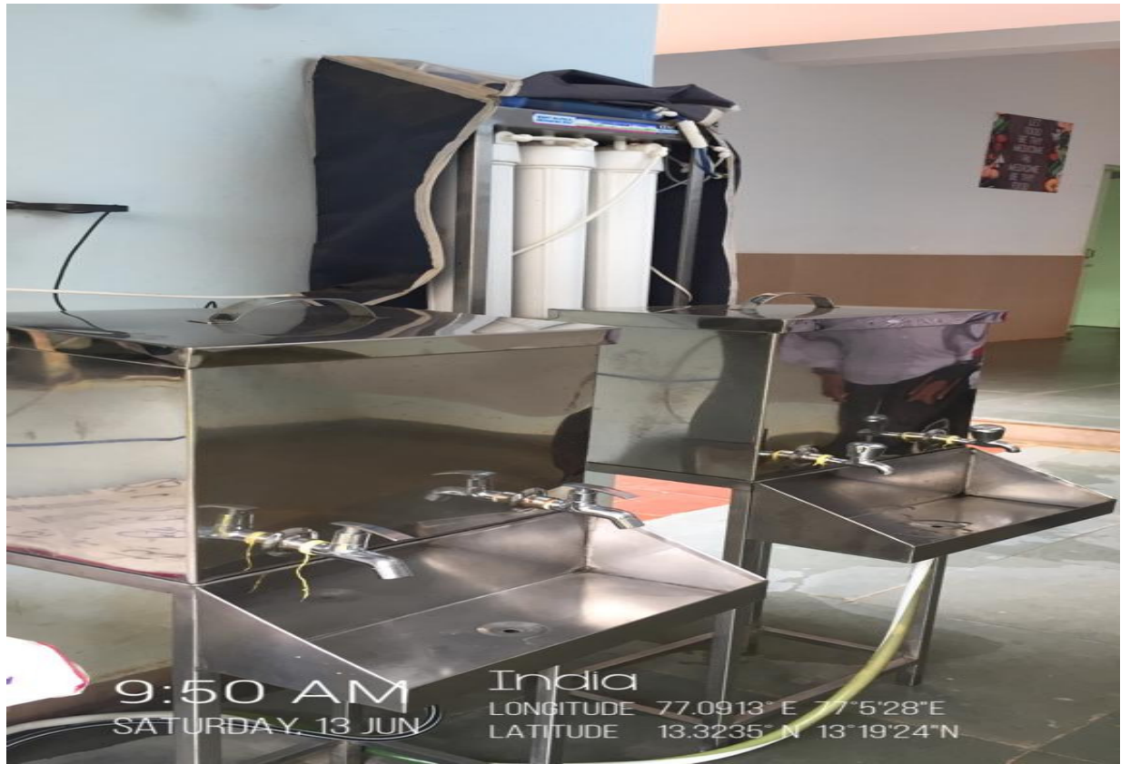
RO drinking water facility in the ladies hostel.
